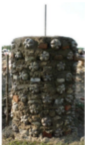
Column in mid-construction. This column was the first that utilized barbed wire for reinforcement.
